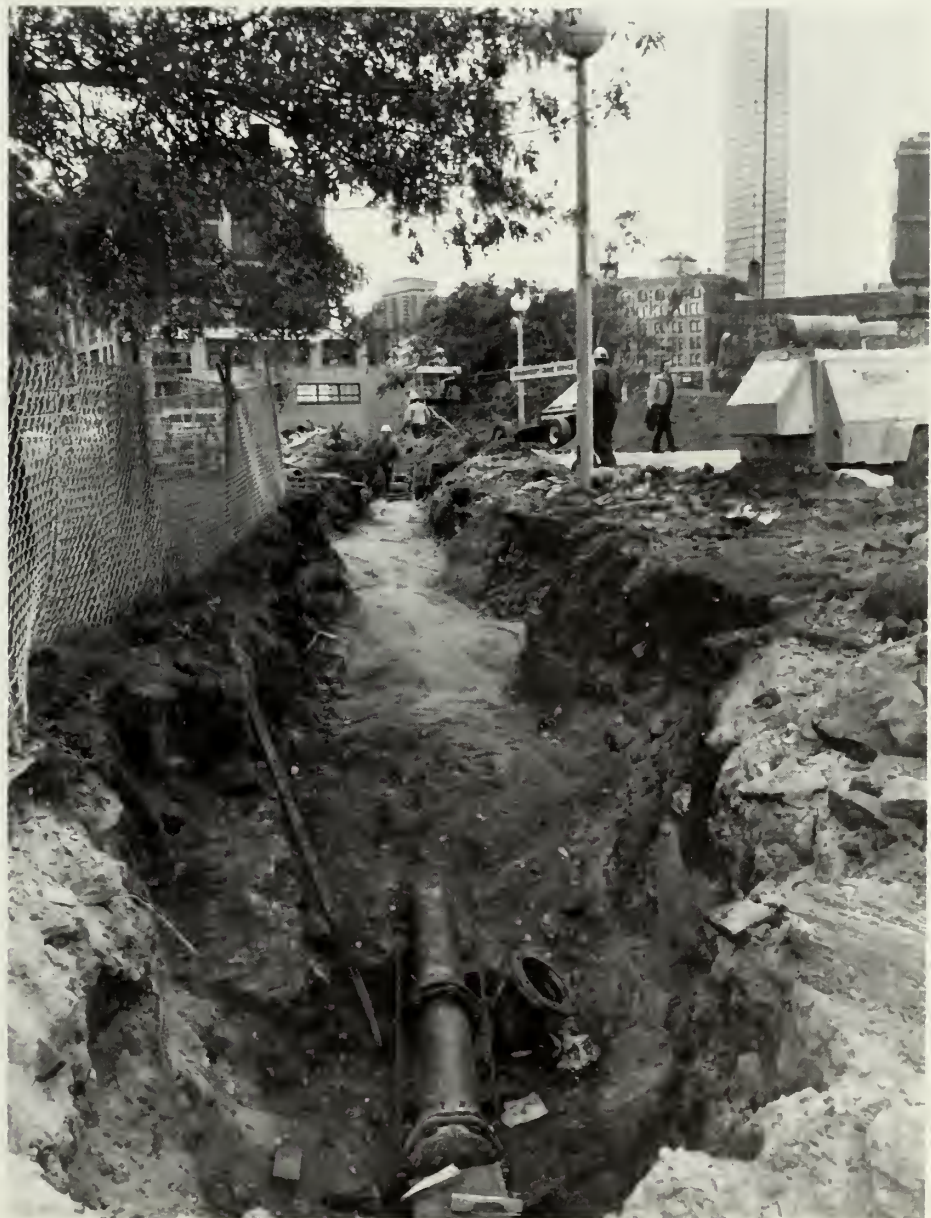
8-INCH WATER MAIN at Chandler Street, Boston, was relocated preparatory to the start of construction of the South Cove Tunnel link between the existing Orange Line and the planned relocated line.
